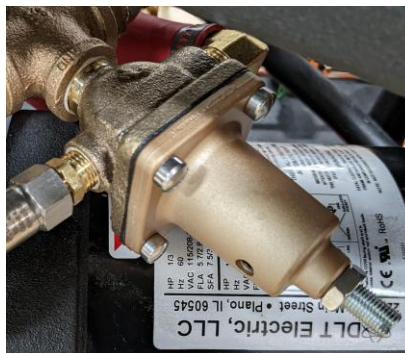
Bypass pressure relief valve
