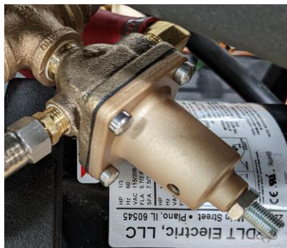
Bypass pressure relief valve, with adjustment post uncovered
